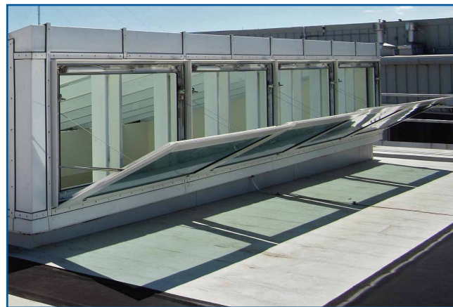
Smoke and Heat Ventilation
